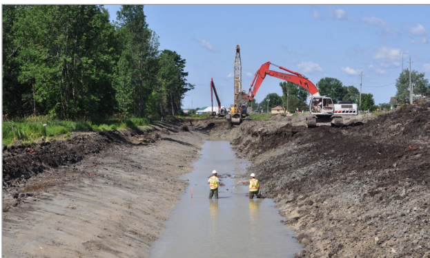
Figure 1. An active drain construction project. Source: Town of Bradford West Gwillimbury, Ontario.
